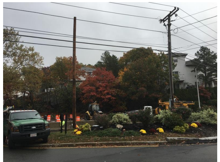
The new utility pole (left) has already been installed. All utilities on the pole on the oval (right) will be moved to the new one
