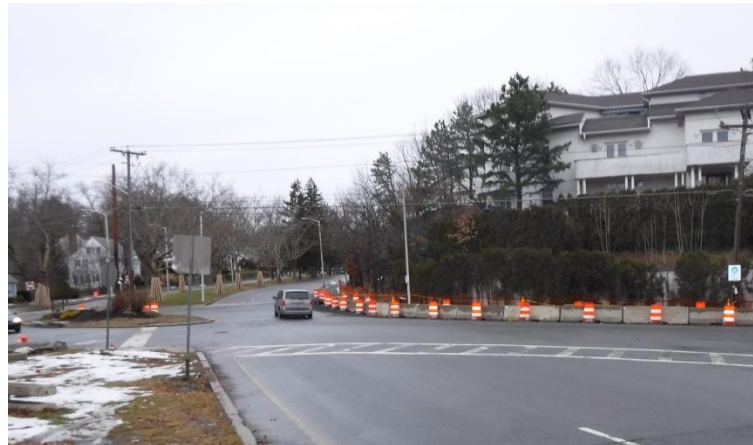
Crews completed excavation for pipes on the northeast corner of the intersection
