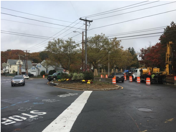
Crews will remove “oval” in the middle of the intersection after the utility companies move their cables off the pole.
