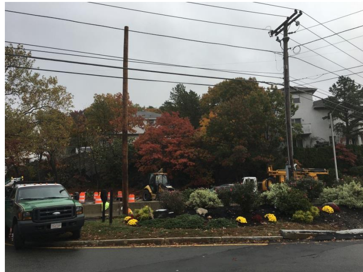
The new pole is to the left in this photo and is off to the side of what will be the new intersection. The old pole is to the right, seen here with all utilities still attached, is in the middle of the “oval.”
